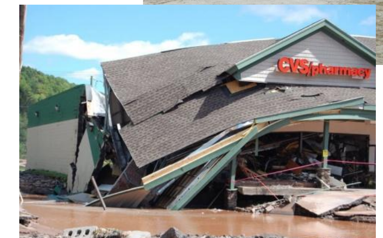
Flooding & damage near CVS/Fresh Town building, 2011
